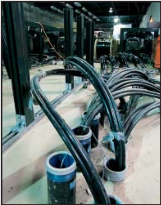
Power and network equipment in Progressive's data center
